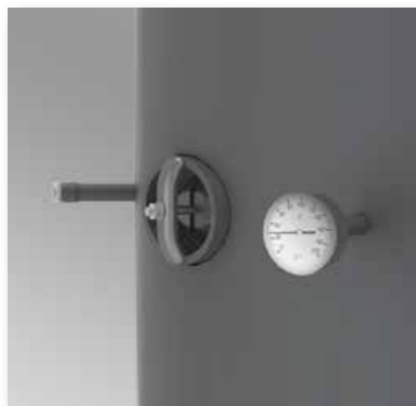
■ Control thermometer and manhole
